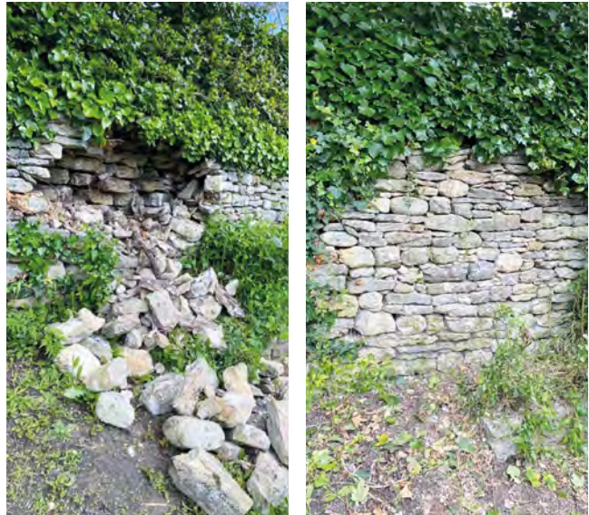
Pictured: a collapsed area of dry stone wall in St Mary's churchyard (left); after mending by expert Peter Mason
