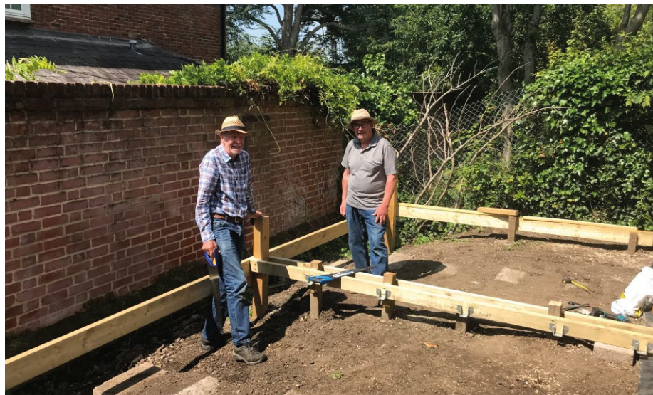
Left: Jim Tigg (left) and Nigel Morgan at work on a new area of decking at the site
